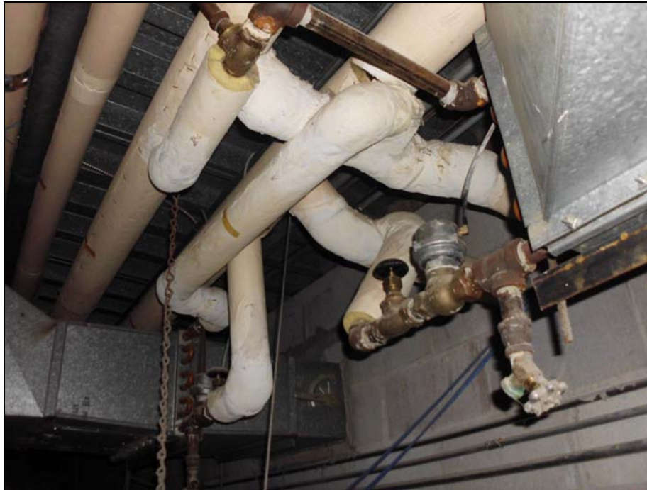
Photograph 3: Asbestos-containing pipe fittings in Corridor 1.C05. Two fittings observed to be in poor condition were repaired in 2011 (Priority 2).
