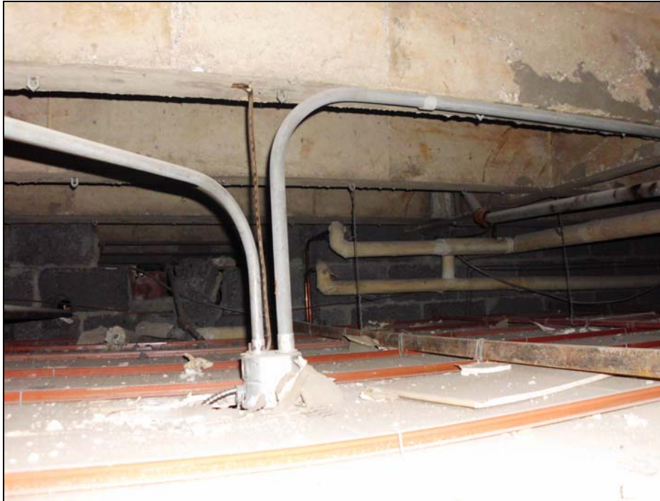
Photograph 1: Asbestos-containing linear pipe insulation and pipe fittings above the suspended solid ceiling in Room 1.31 – Girls Washroom. Pipe fittings identified as Priority 1's were repaired in 2011.
