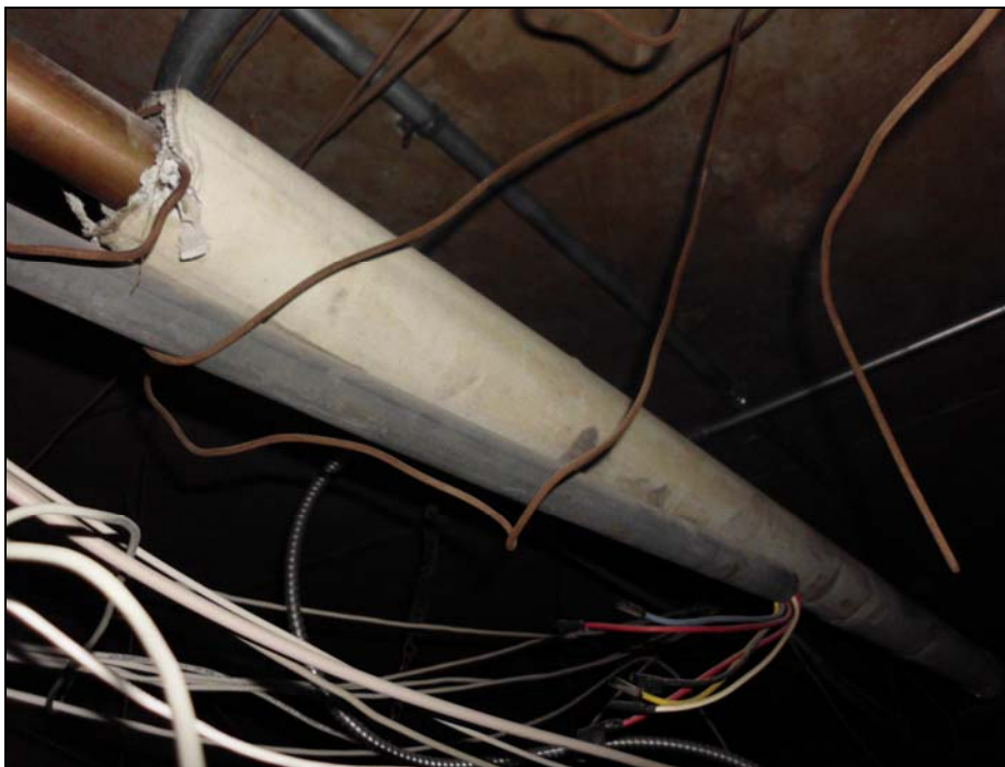
Photograph 2: Asbestos-containing AirCell pipe insulation with exposed ends in Corridor 1.C02 was removed in 2011.
