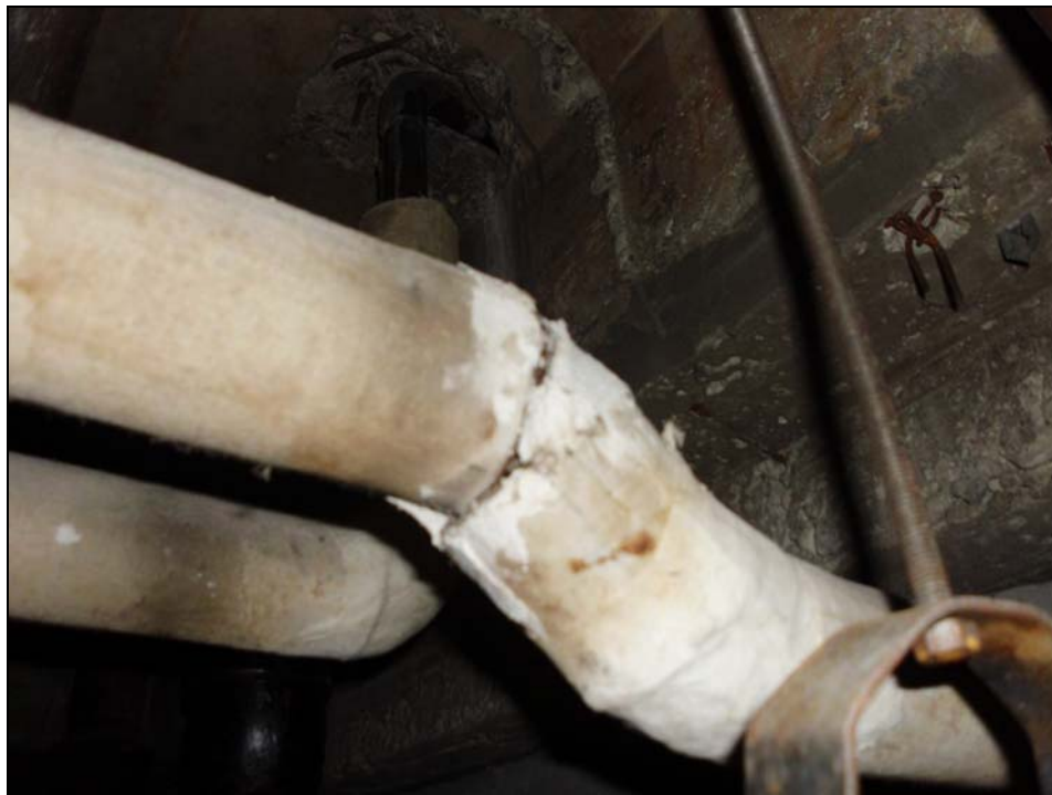
Photograph 4: Asbestos-containing pipe fittings above the suspended solid ceiling in Room 1.31 – Girls Washroom. Three fittings were observed to be in poor condition and were repaired in 2011 (Priority 2).
