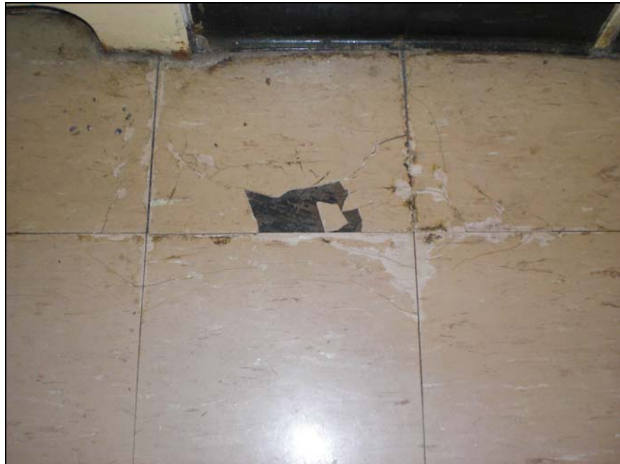
Photograph 5: Assumed asbestos-containing vinyl floor tiles in poor condition in Room 1.09 – Classroom were repaired in 2011 (Priority 2).
